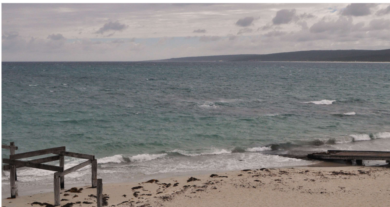
Hamelin Bay looking north: old jetty on left, ramp on right (K Klaka)
