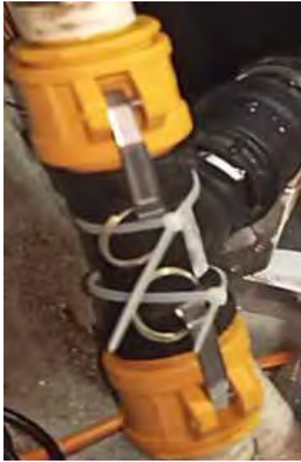
Cable ties hold the fitting closed
